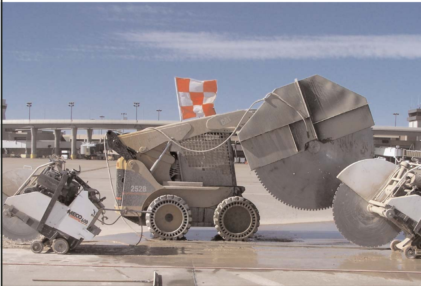
Flat saws were used with varying diameters to cut the perimeter of Taxiway K at DFW International Airport.
