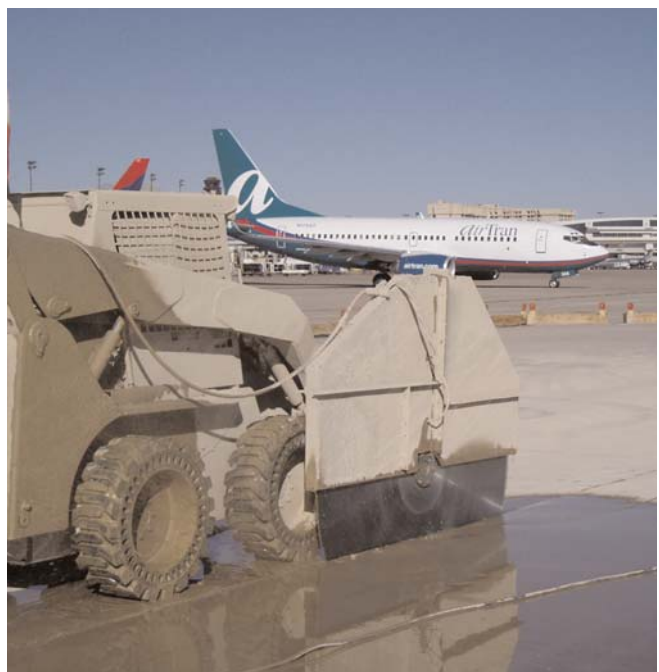
Airport operations continued as usual while workers cut the perimeter of Taxiway K.
