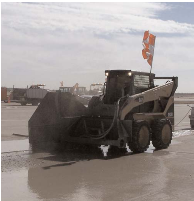
Workers cut in different stages in order to achieve the required depth of 41 inches.
